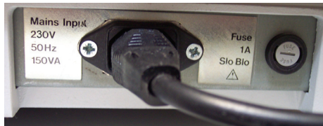
Figure 12 Mains connection and voltage plate
